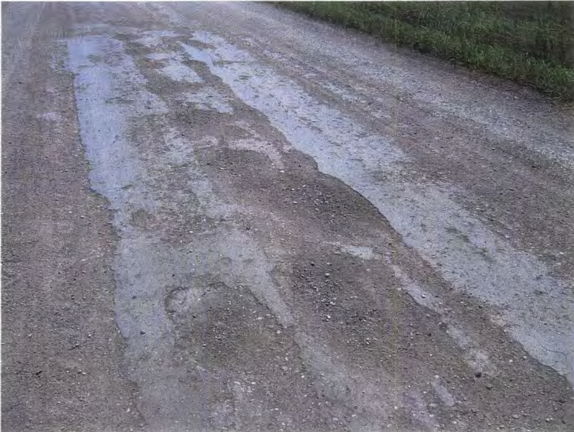
Figure 6.2.5. Centerline potholes in the soapstock on Grant Avenue.
